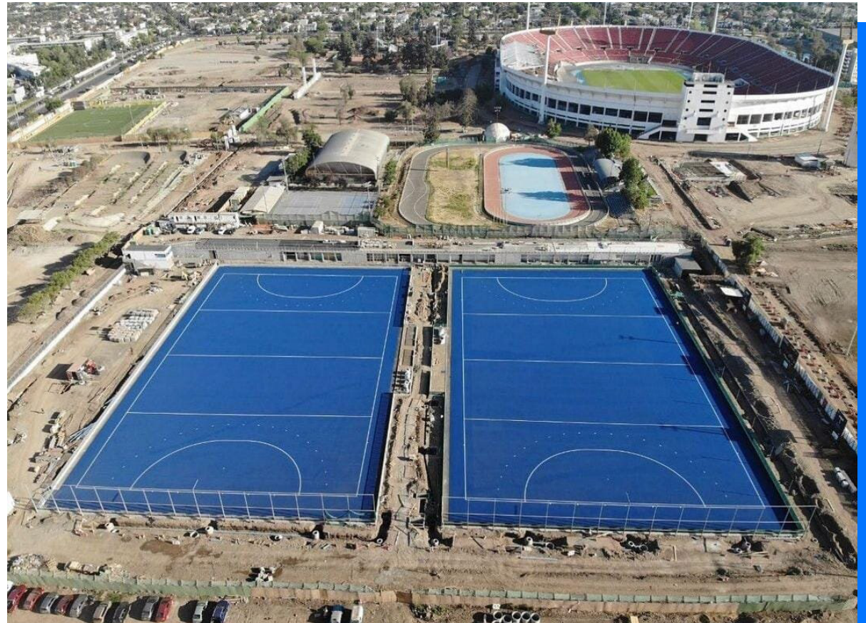
This is how the public Field Hockey fields will look like, currently under construction at the National Stadium Sports Park.
